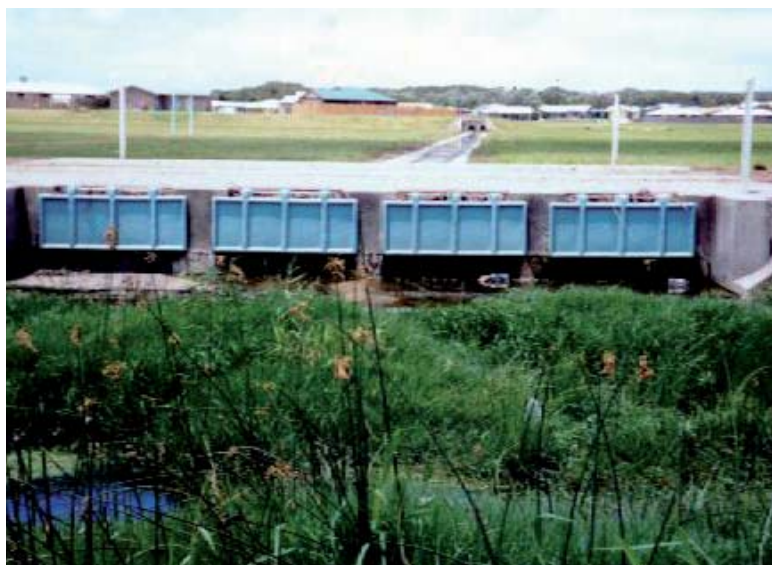
4 x 1200 x 375 installed at Eagle Mount Heights, Mackay, Qld
